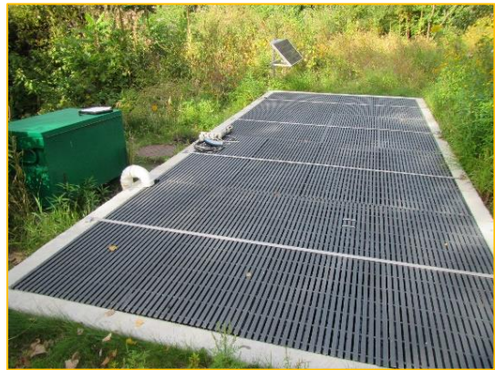
Figure 30 Spent Lime Treatment System
