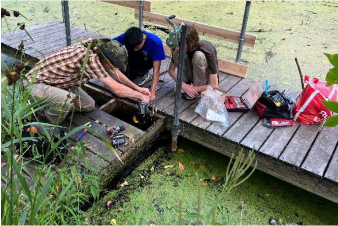
In 2022, a teacher from Scenic Heights Elementary utilized an Educator Mini-Grant to purchase materials to repair a dock at a pond on school property. Students can now access the pond more safely to learn about water resources.
