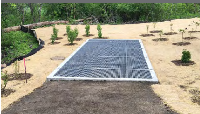
Figure 57. Spent Lime Treatment System
