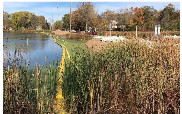
A double row of yellow silt curtains in the water protect the lake from the Duck Lake Road construction zone (fall 2021).
