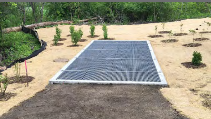
Figure 57. Spent Lime Treatment System
