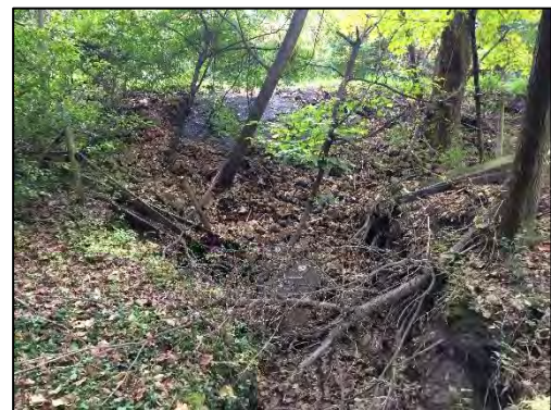
Eroded ravine downstream of road drainage
