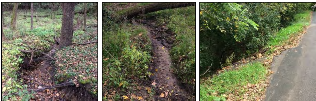
A. Ravine erosion at upstream end near Pleasantview Road B. Ravine erosion at downstream end near Silver Lake C. Low spot along Pleasantview Road where runoff enters ravine Figure 2-4 Ravine Erosion
